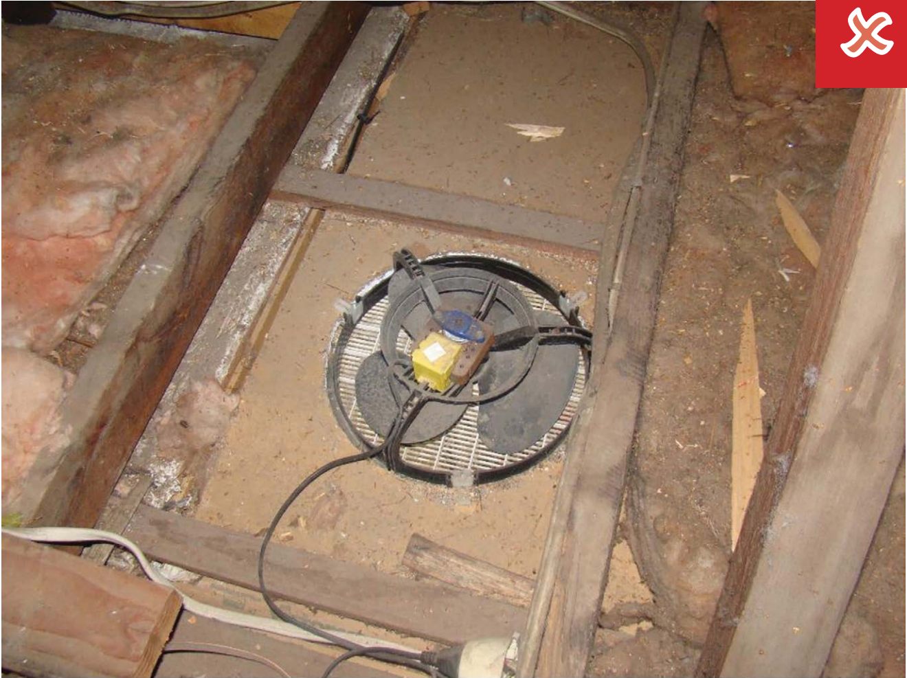
Figure 6. Poor installation practice
