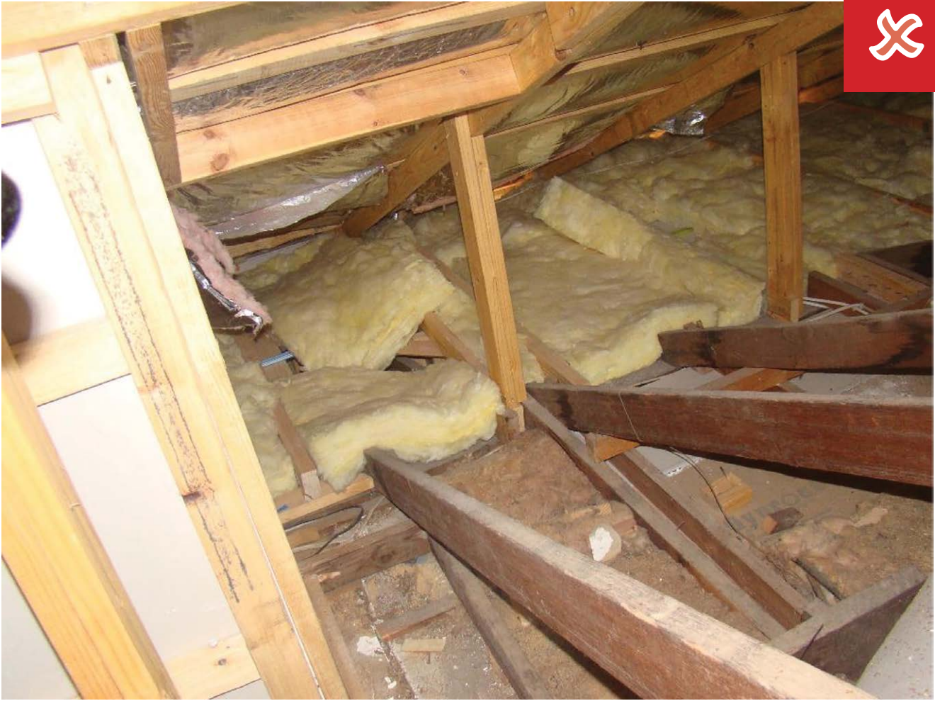
Figure 5. Poor installation practice
