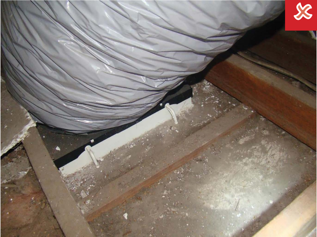
Figure 4. Poor installation practice
