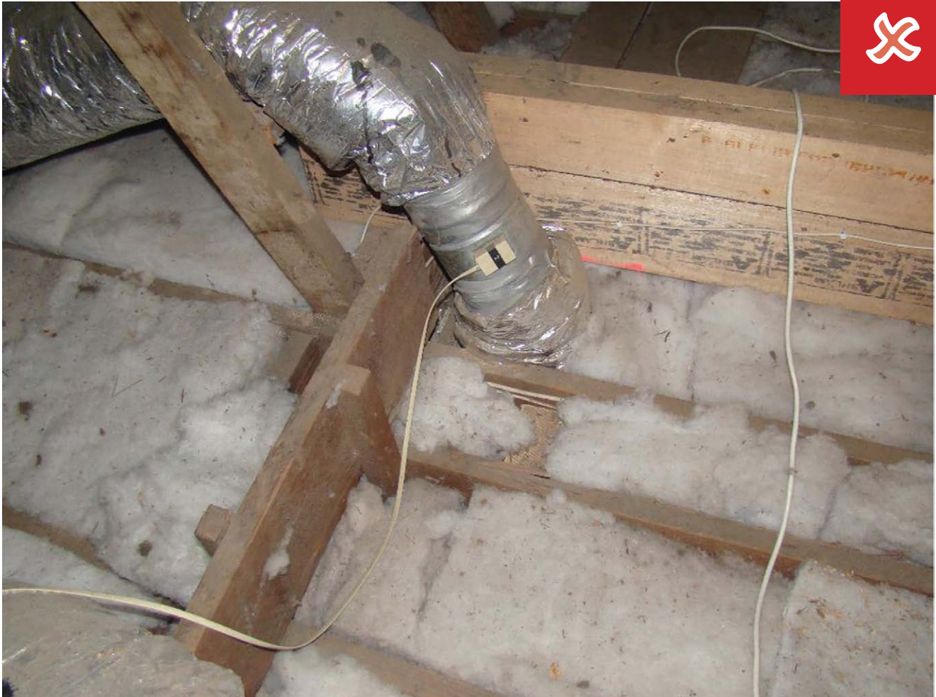
Figure 3. Poor installation practice
