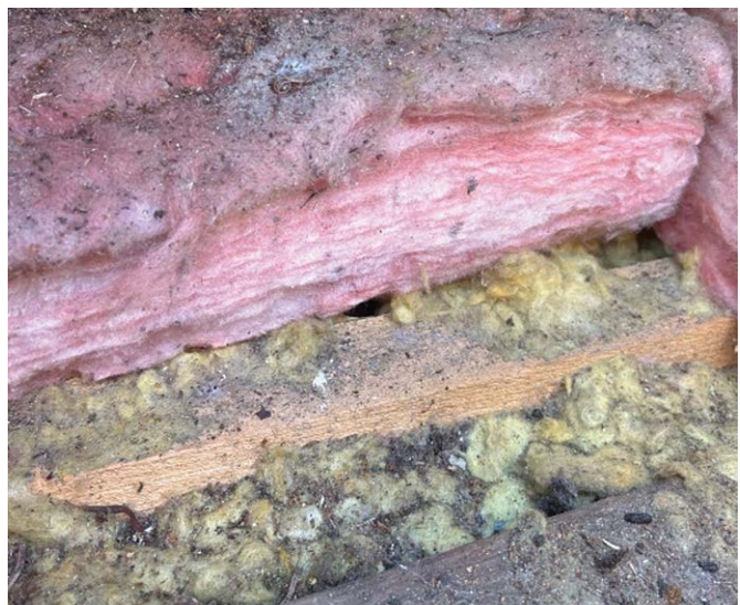
Figure 1. Multiple layers of insulation materials
